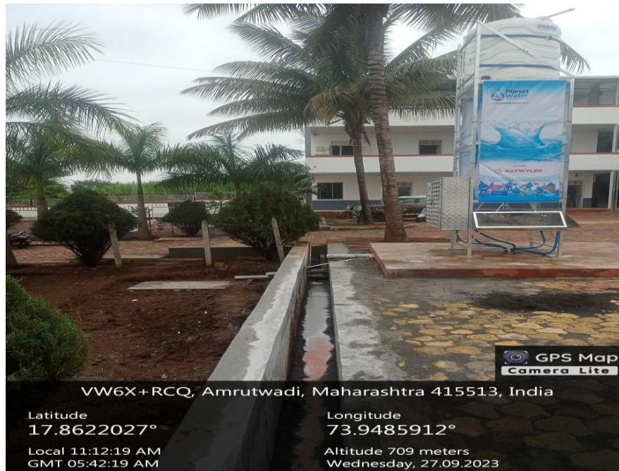
Water Purifier System
